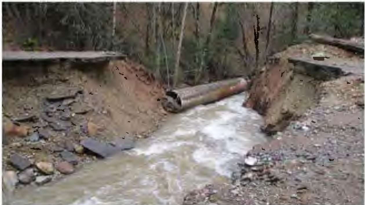
Figure 4-107 Plumas County – Thompson Creek Washout
