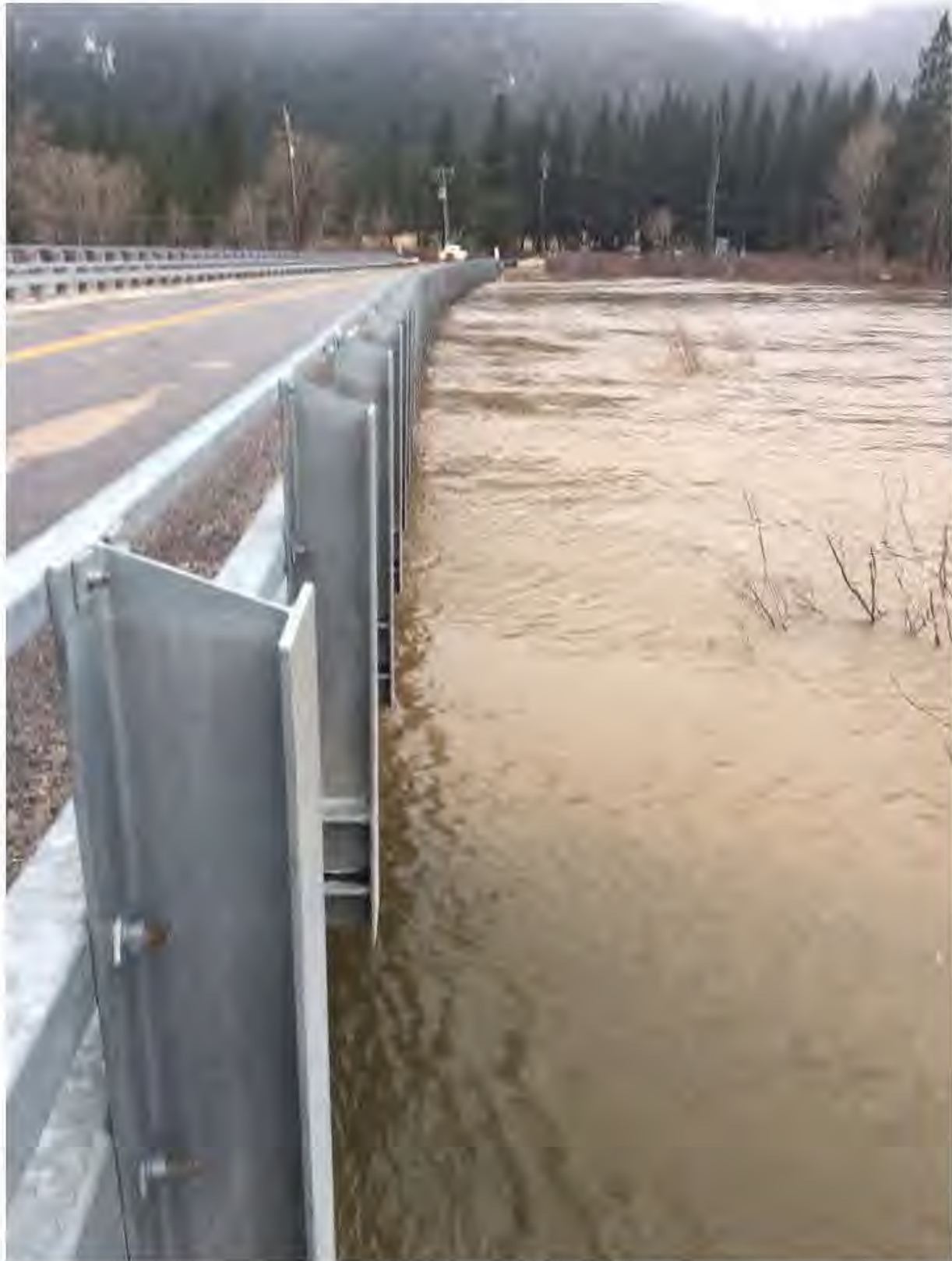
Figure 4-102 2017 Flooding – Arlington Bridge
