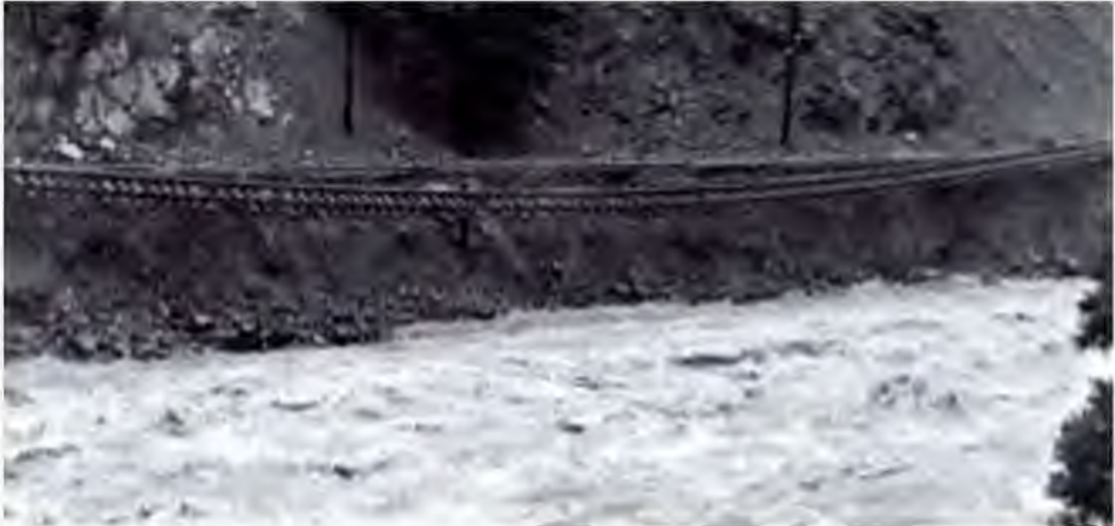
Figure 4-92 1986 Railroad Bed Flood Damages
