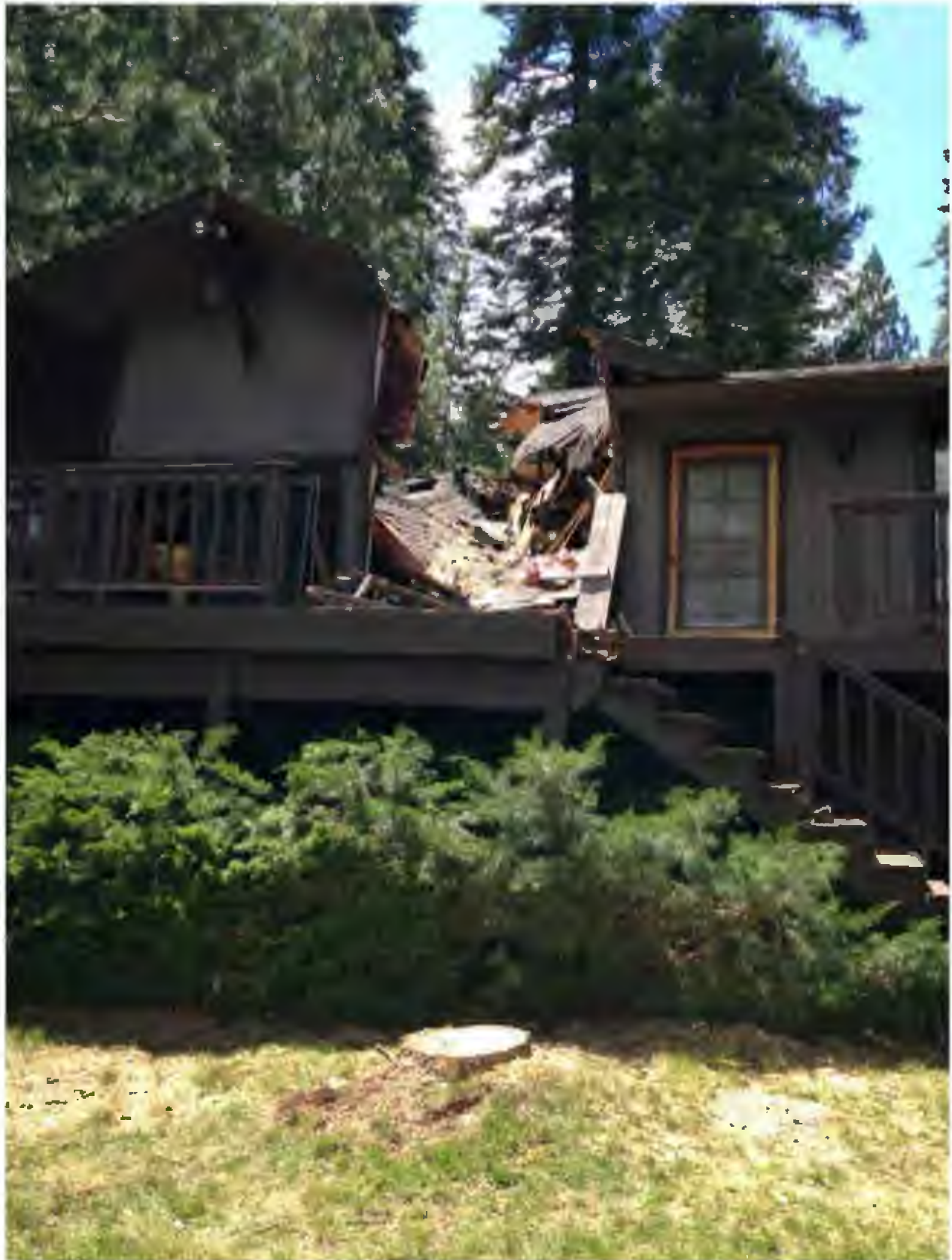
Figure 4-29 Plumas County – 2015 Wind Event Damage
