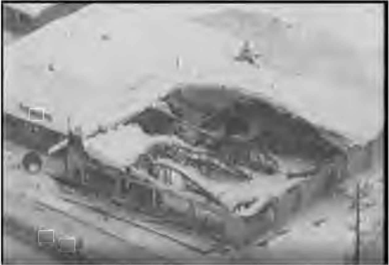
Figure 4-38 1993 Storm Damage of Store in Quincy
