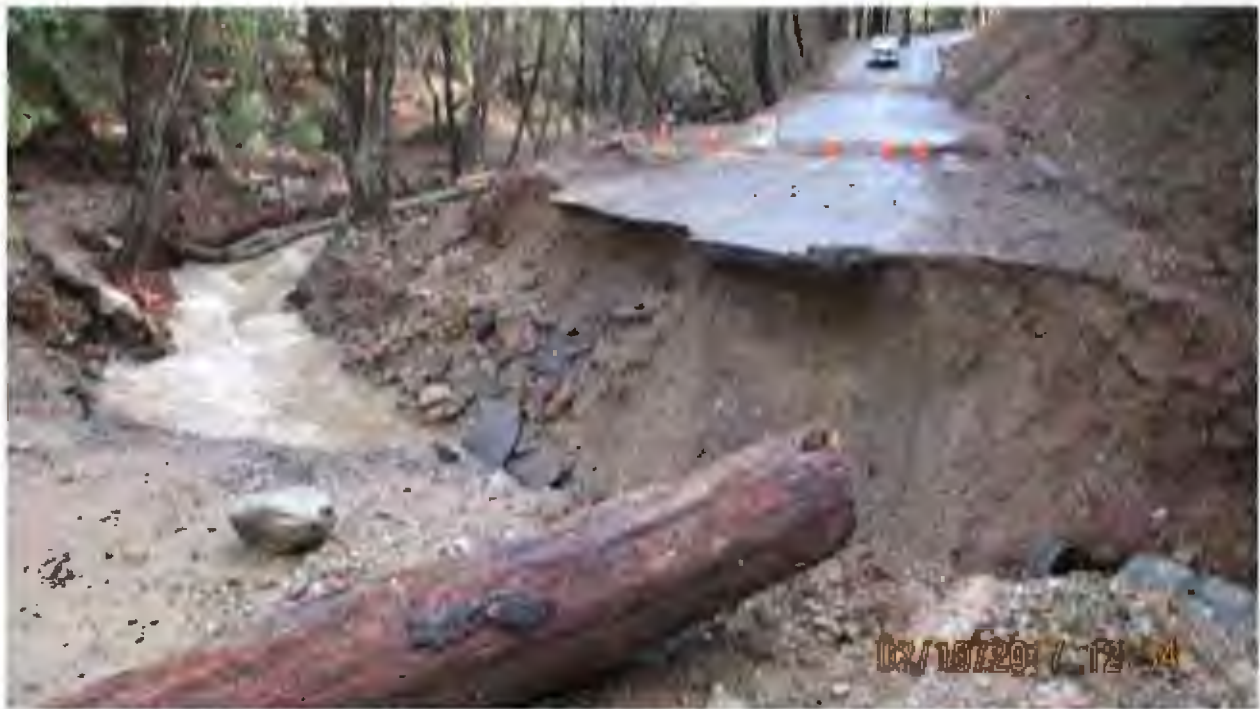
Figure 4-106 Plumas County – LaPorte Road Washout
