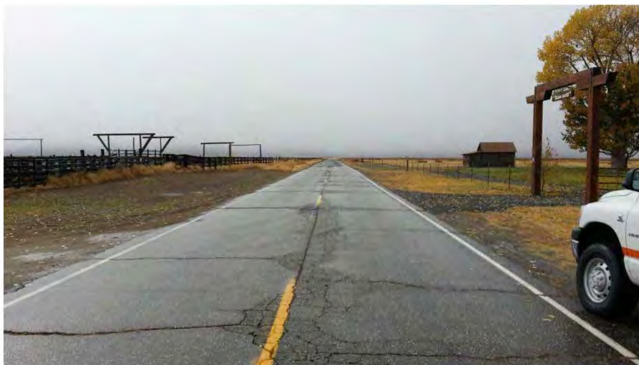
Figure 4-117 Harriet Lane – Pavement Deterioration from Localized Flooding
